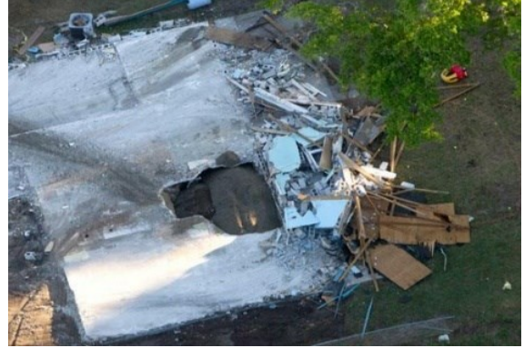
Figure 1.3 An aerial view of the sinkhole which was exposed after the house was demolished, Seffner, Florida (Morel, 2013)
