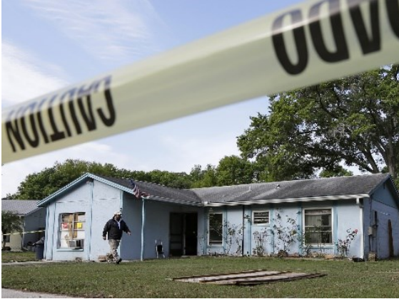
Figure 1.2 An engineer surveys in front of the home where a sinkhole opened up in Seffner, Florida (Memcott, 2013)
