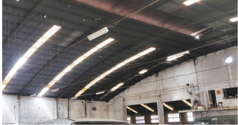
Photograph of steel truss curved roof structure of the warehouse typology in the area.
