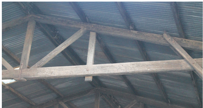
Photograph of timber gable roof structure of the warehouse typology in the area.
