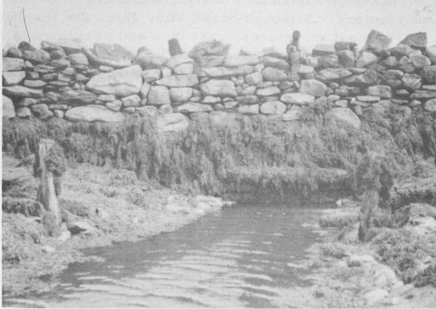
Fig. 5 - An aboiteau located in Yarmouth County which was built many years ago. The lower half of this structure was made with quarried rock and a steel gate was hung over the sluice exit which cannot be seen in this photograph.
