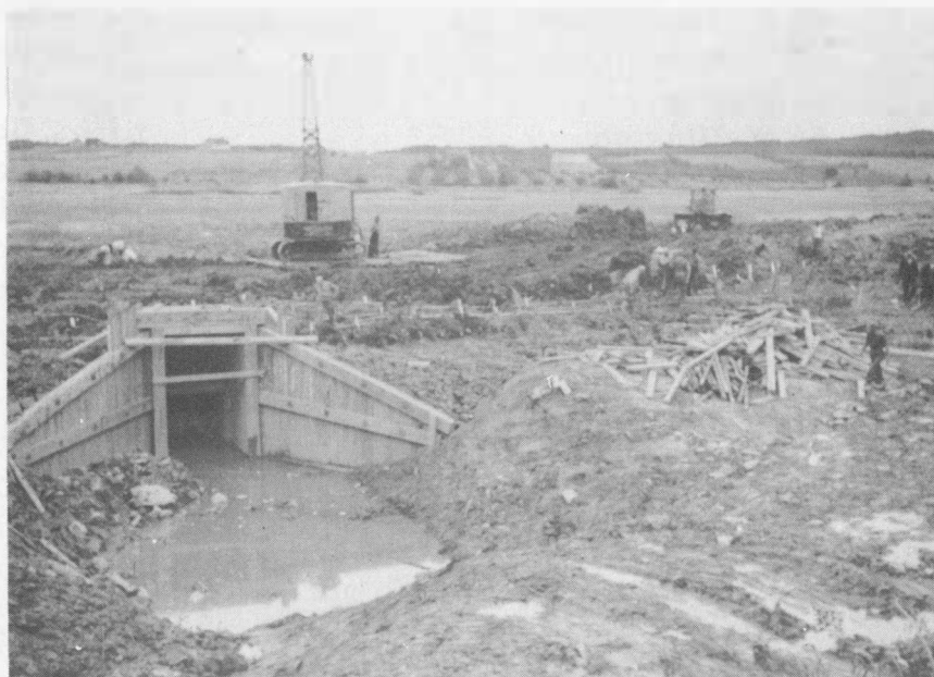
Fig. 12 - This photograph shows the placing of fill and brush in the structure which is to replace that shown in Fig. 11. The downstream porch, wingwalls and sluice end may be seen.
