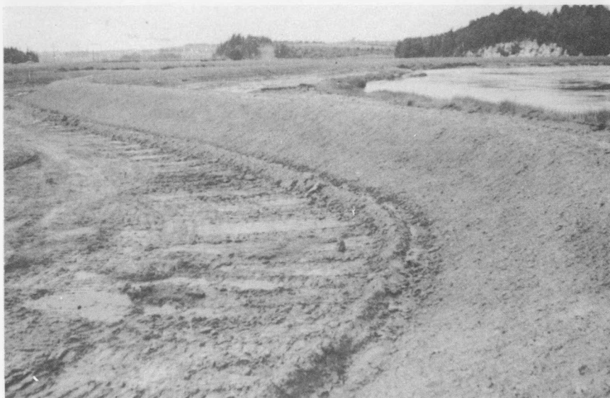
Fig. 2 - A new constructed up-river dyke near Brooklyn, N. S. Bulldozers and a grader were used. The new dyke, at some locations is behind the old dyke.
