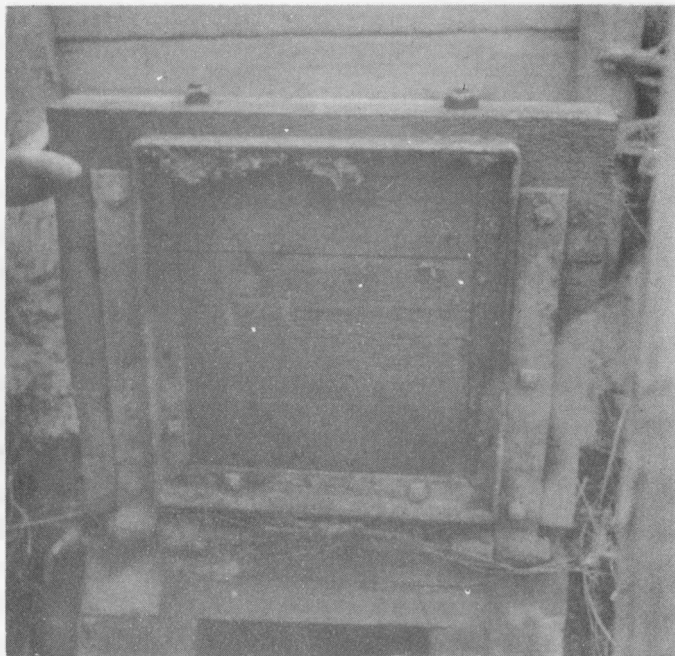
Fig. 14 - This photograph shows the gate on the sluice indicated in Fig. 13. The angle iron on the gate was placed in an attempt to prevent leakage of salt water and silt. However, this was not satisfactory. This aboiteau sluice was built many years ago.
