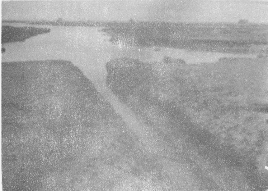
Fig. 20 - This is a photograph of marsh out to tide near Amherst, N. S. In the immediate foreground is what was once a small field drainage ditch and this continued well into the background. The tide flowing on and off the marsh has eroded this ditch at the rate of about 1000' per year.
