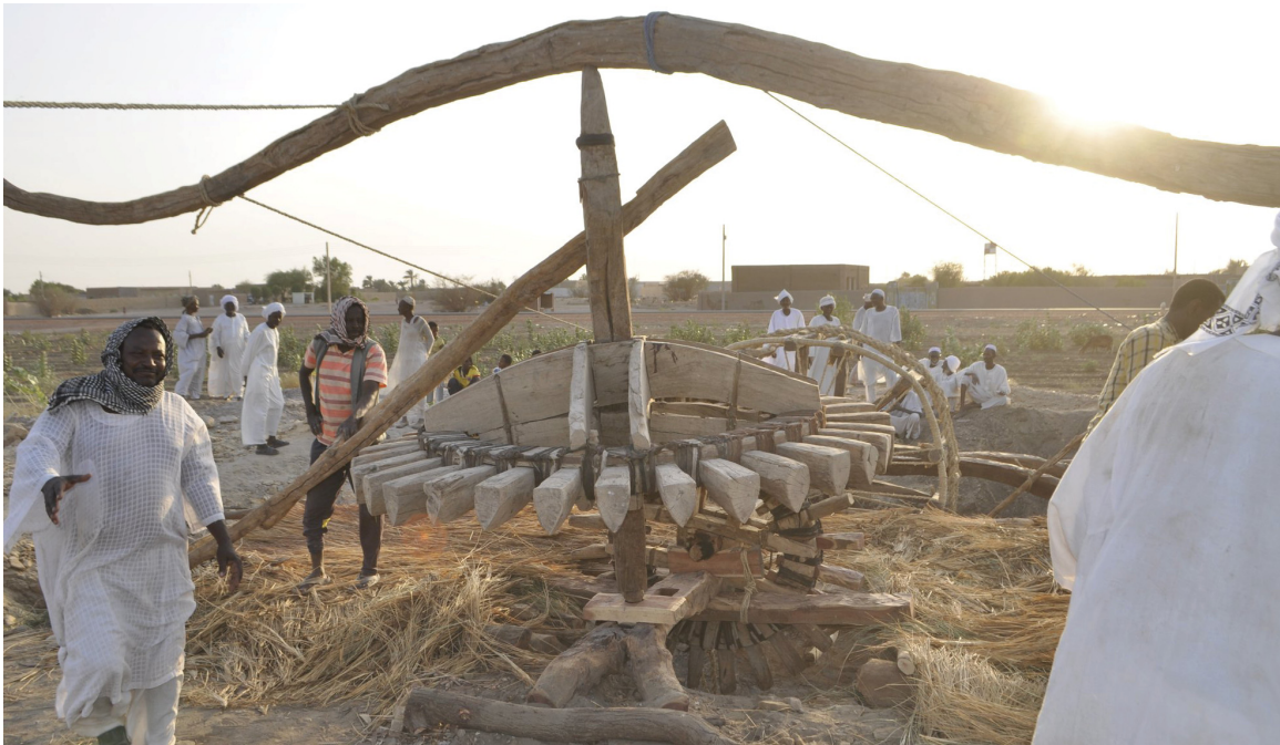
A modern saqiya undergoing final stages of construction (National Council for Culture Heritage and the Promotion of National Language n.d.)
