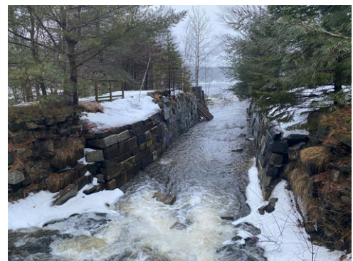
Figure 37: Location D - Lock 4 overflow
