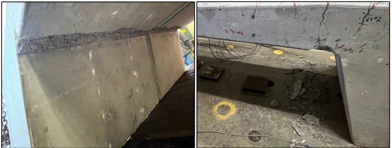
Figure 4-26. Rehabilitation Specimen Ultimate Failure Concrete Crush
