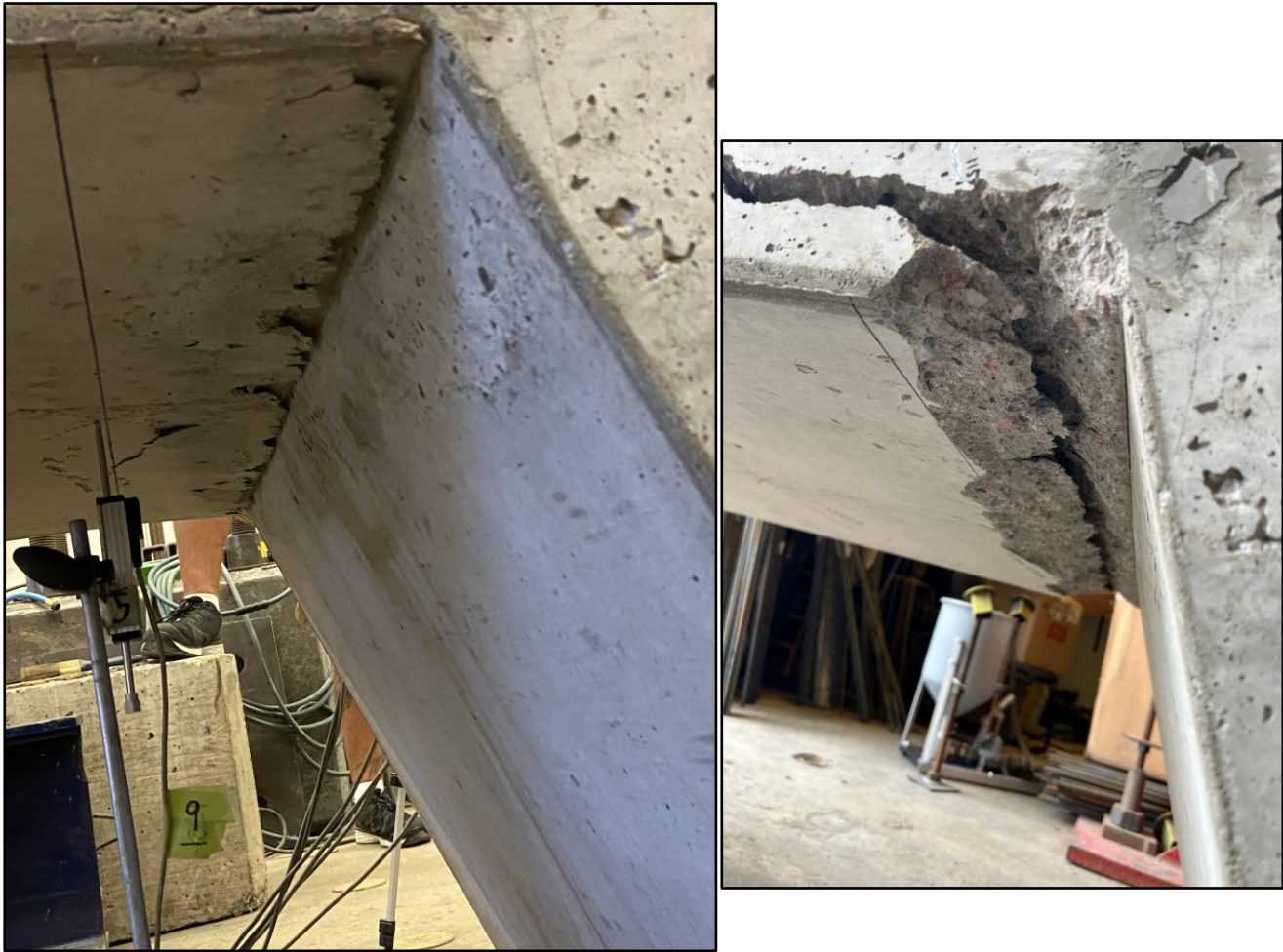
Figure 4-18. Control Specimen Ultimate Failure Concrete Crush
