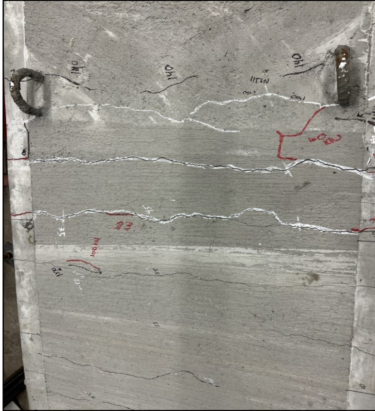
Figure 4-15. Control Specimen Top Slab Cracking Pattern
