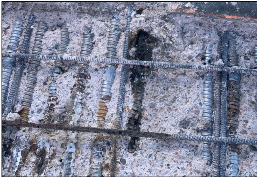
Figure 1-1. Corroded Transverse Steel Post-Tensioning (photo taken by Faraj Shahrstan in 2020)
