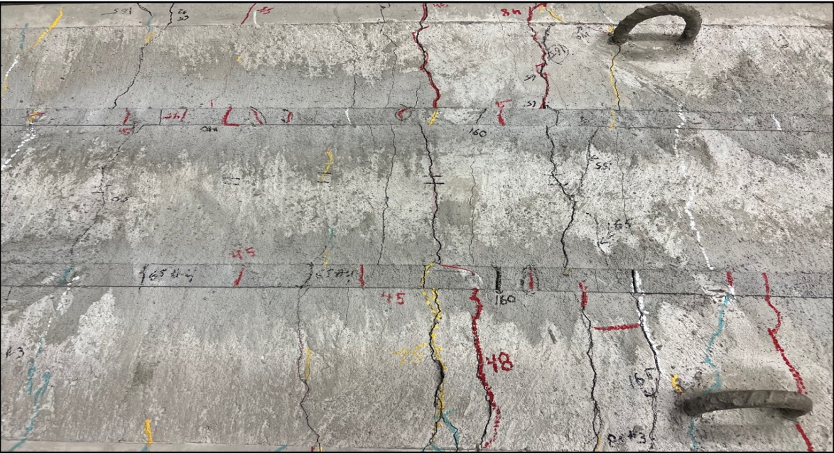
Figure 4-22. Rehabilitation Specimen Top Slab Cracking Pattern
