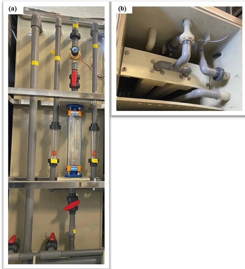
Figure 3.1 (a) Exterior view and (b) interior view of the membrane tank
