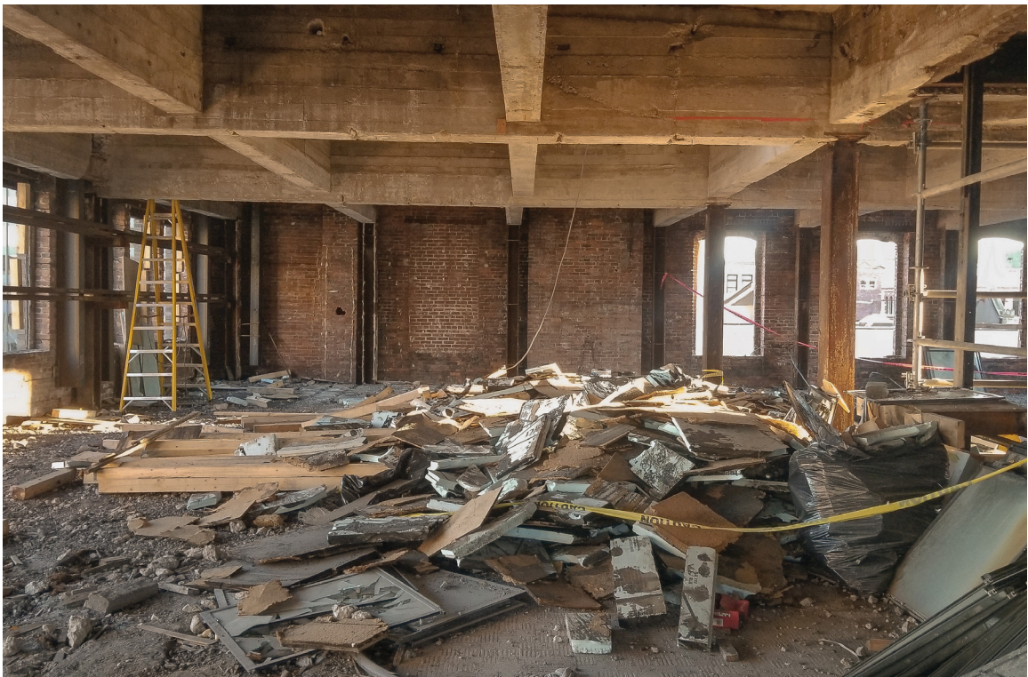
Unsalvageable material at demolition site on Granville St. and George St.
