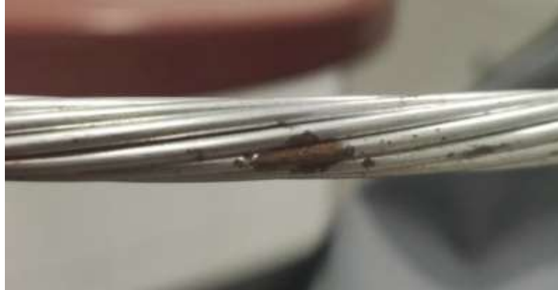
Figure 10: Localized corrosion spot on bead strand
