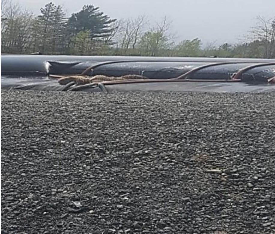
Figure 8. Pilot Geotube® de-watering system located just outside the Boat Harbour Aeration Stabilization Basin.
