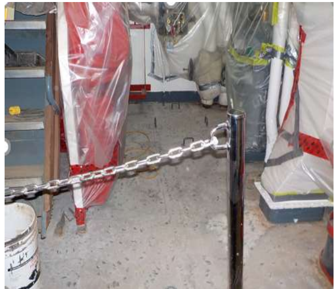
Figure 6: Deck work generally makes all nearby equipment inaccessible.
