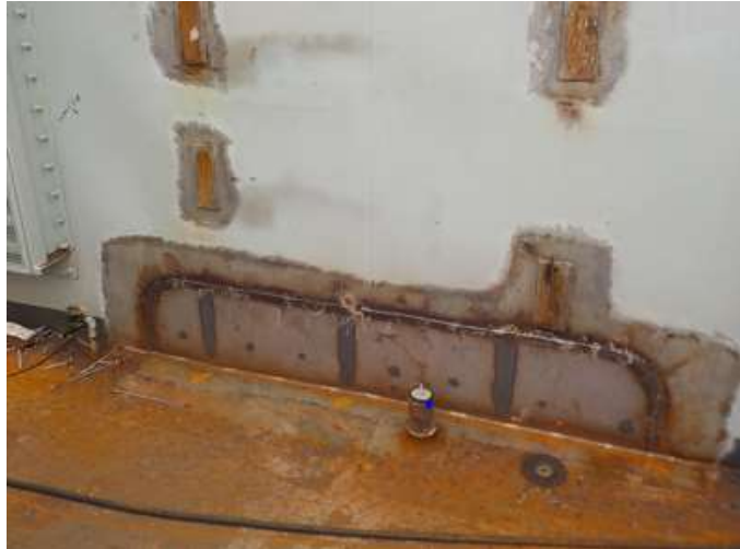
Figure 8: Hot work on this corner affects three adjacent spaces, placing them out-of-bounds.
