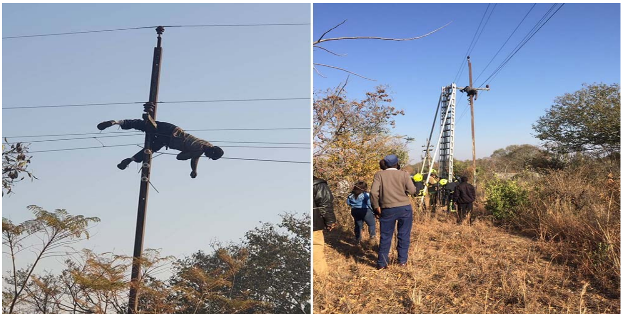
Figure 4. 3 The Fiery end: A copper cables thief was electrocuted when the power came back on (Pic: Lenin Ndebele, 2019)
