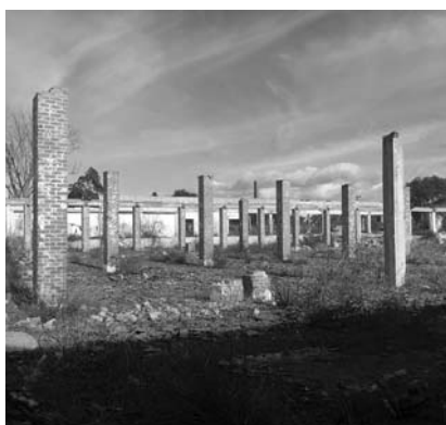
Figure 72 (top): View of tiling pattern on vernacular building Figure 73 (bottom): View of warehouse columns in a state of ruin
