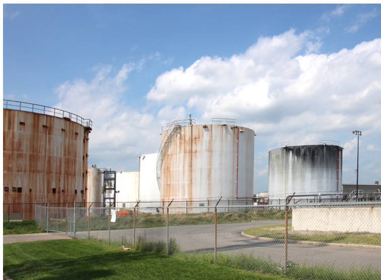
Oil storage tanks at base of Pier 12, showing age and large scale change in industrial zone, 2018.
