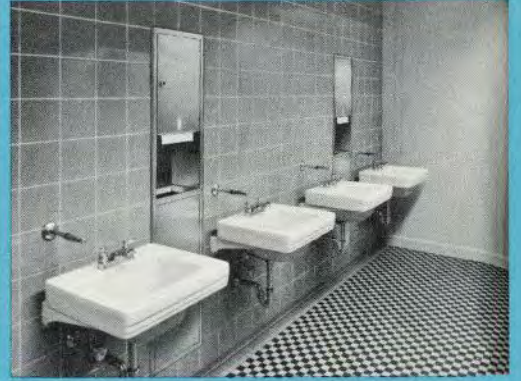
Typical Washroom Installation
