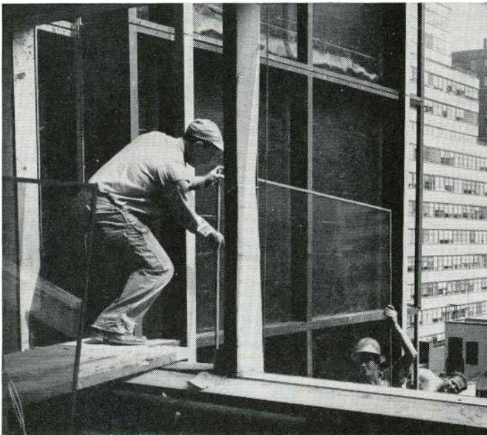
Glass light being lifted into place. Neoprene gasketed edges make lights easier, safer to handle.
