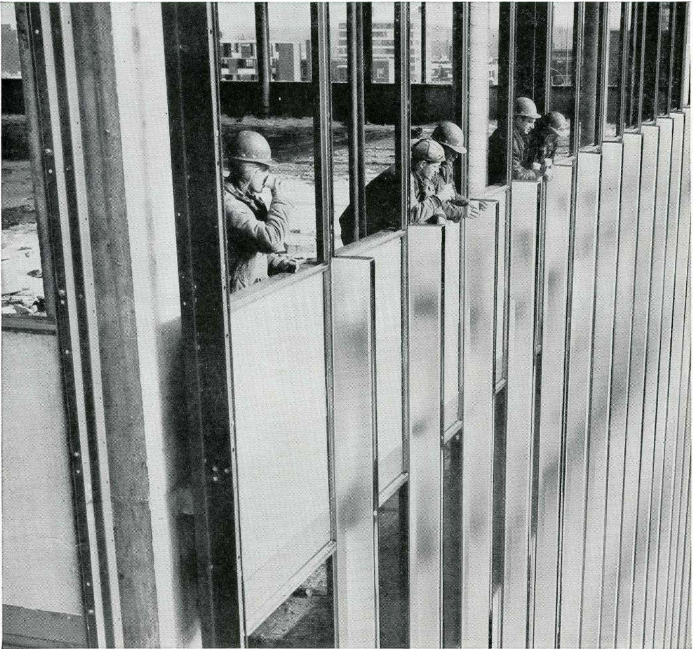
Stainless curtain wall erection, 130 Bloor Street West, Toronto. Architects: Bregman & Hamann. Contractor: Perini Ltd. Owner: Cemp Investments Ltd.
