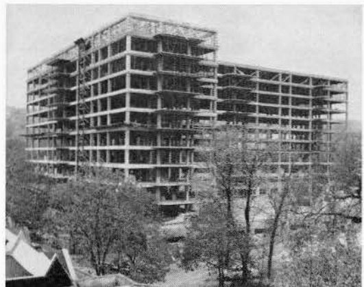
Structure: The Forty-Three Hundred, Westmount, Que. Architect: Ian Martin Consulting Architect: Maxwell M. Kalman Structural Engineer: Irving S. Backler General Contractor: Louis Donolo Inc.
