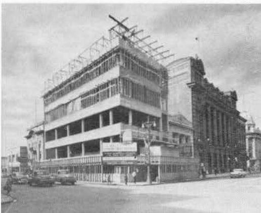
Structure: The Huron and Erie Corporation and The Canada Trust Company Building, Winnipeg, Man. Architects and Engineers: Moody and Moore Contractor: Commonwealth Construction Co. Ltd.
