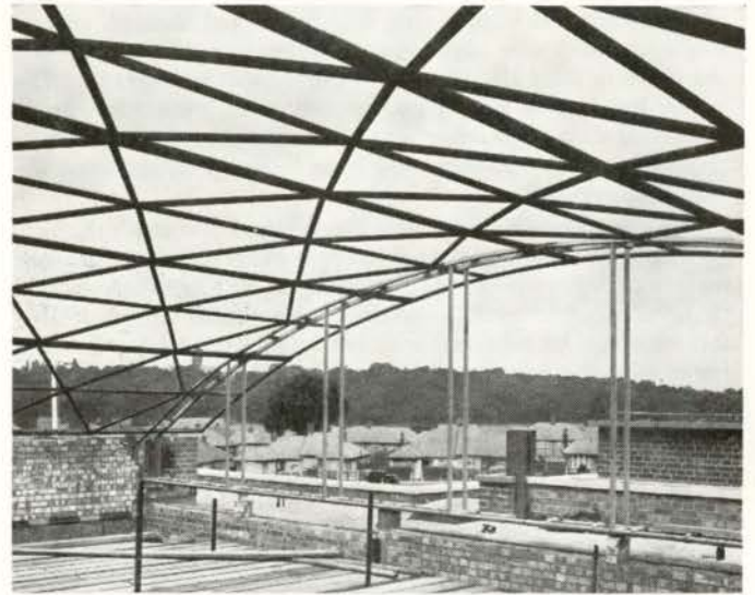
Fig. 7 The Gilbert Colvin School for Ilford Borough Council. Tubular steel space frame by Ove N. Arup and Partners, consulting engineers in conjunction with Scaffolding (Great Britain) Ltd.
