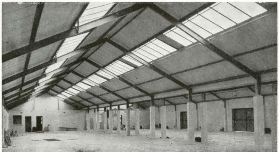
Fig. 2 Store building, Rosyth, designed by the plastic design method. Royal Naval official photograph, published by permission of the Admiralty.
