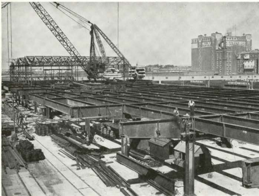
Fig. 3 Transit shed for passengers and cargo, Southampton. Designed by the plastic design method. Consulting engineers: Scott and Wilson, Kirkpatrick and Partners.
