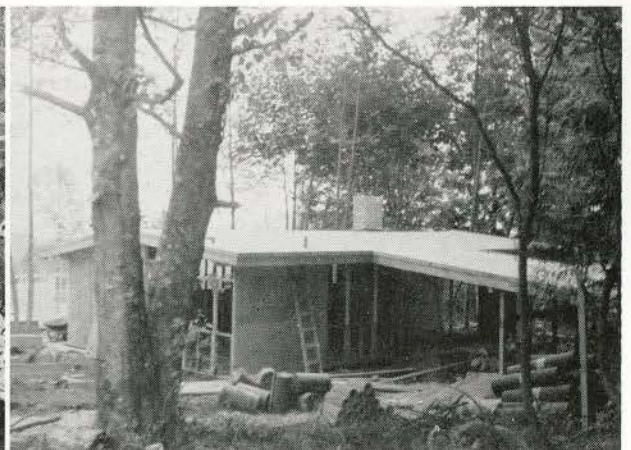
Development House: One of two houses designed and constructed by three third year students—Ron Nelson, Gordon Hartley, and George Barnes—who incorporated themselves into Timberline Homes Company Ltd. during the summer of 1954. These students propose to continue this venture during further summers.
