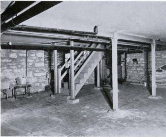
BEFORE —Here's a typical basement, damp and unhealthy, because hard rains seep right through the walls.
