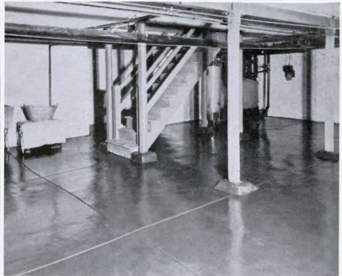
AFTER —Treated with Bondex Waterproof Cement Paint, the same basement is bone-dry and ideal for laundry work.
