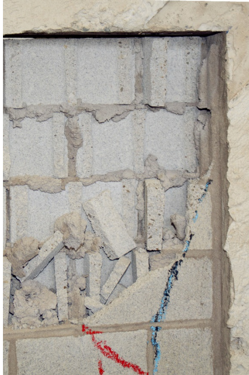
Figure 4.29 Web Shear Failure of Masonry Units for Specimen IF-RC-TG
