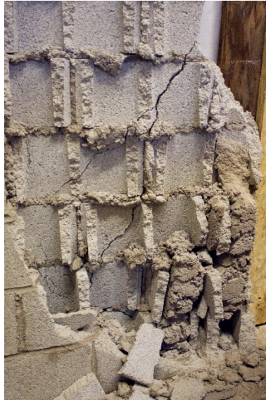
Figure 4.12 Web Shear Failure of Masonry Units for Specimen IF-RC-DO
