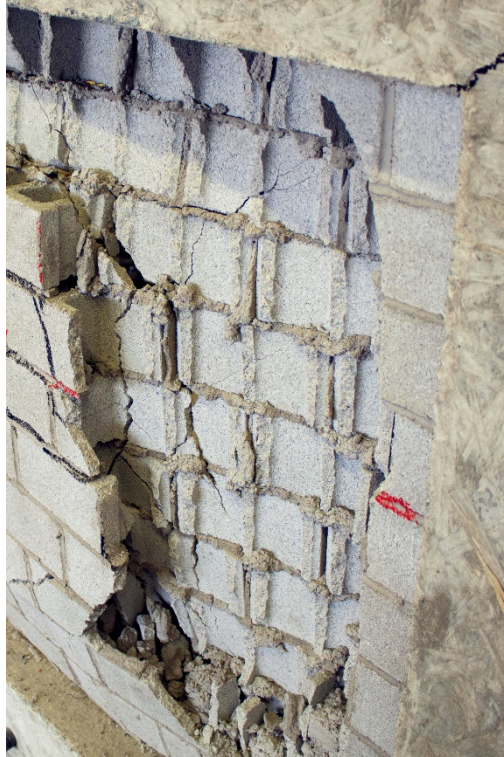
Figure 4.23 Web Shear Failure of Masonry Units for Specimen IF-RC-ID
