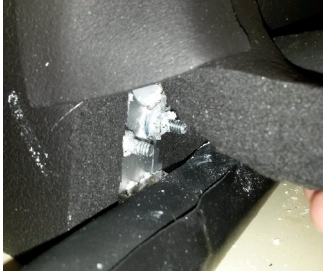
Figure 3-30: Evidence of an SAT leakage source along a compression bolt in the Mark II heat storage cell, shown encrusted with sodium acetate solid (either anhydrous or trihydrate). The appearance of this containment breach corresponds with the appearance of trace solid in Figure 3-29.
