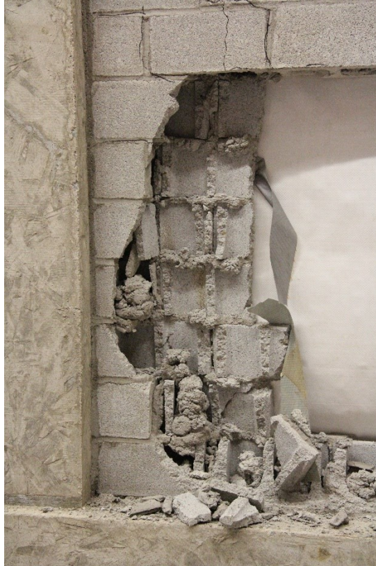
Figure 4.19 Web Shear Failure of Masonry Units
