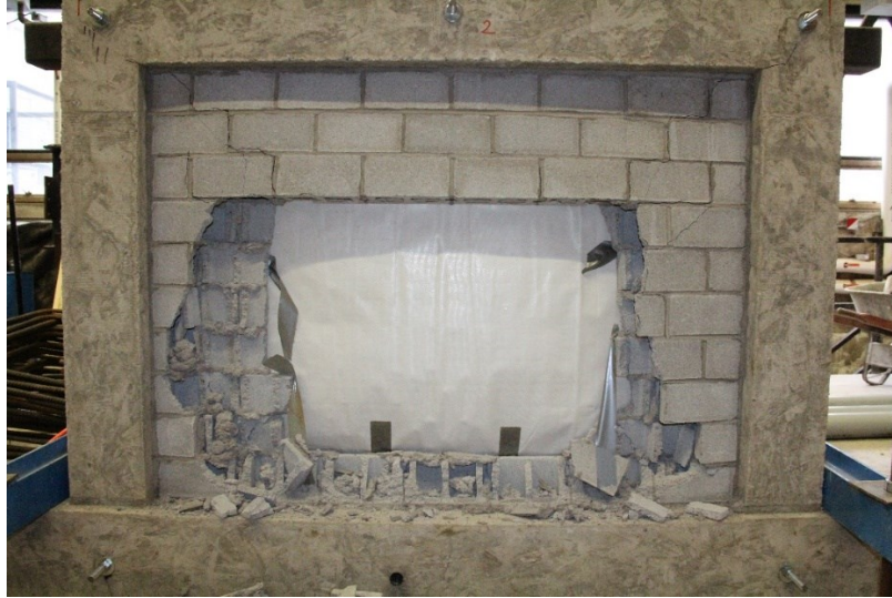
Figure 4.17 Failure Mode of Specimen IF-W-ND
