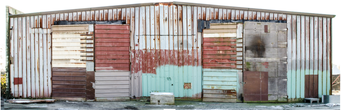
Figure 52: Current Wilkinson Warehouse Building with new roof which shows the historical conservation agenda
