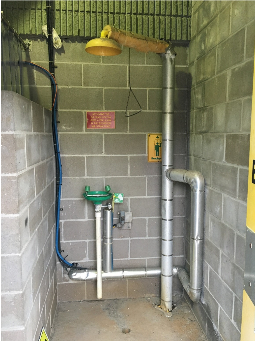
Safety shower and eyewash station located inside yellow door labeled 'PUSH EMERGENCY SHOWER'
