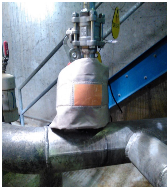
Figure 3 - Chemical leak indicator wrap found on point of acid injection into WAS line.
