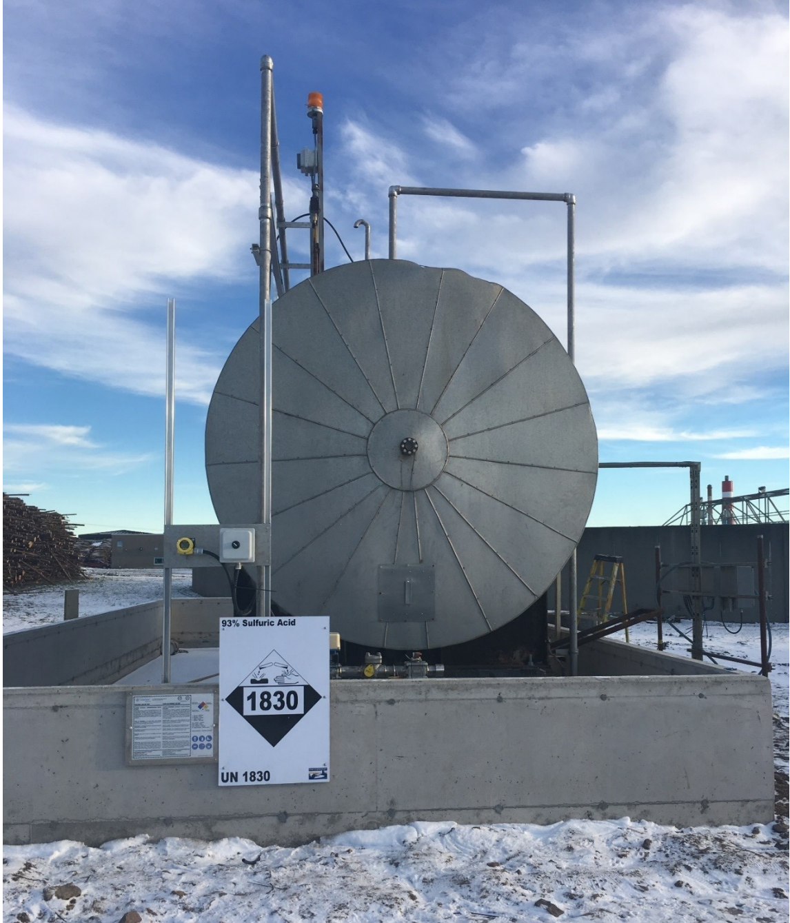
Sulfuric Acid unloading area is located on the north side of the tank as pictured above.
