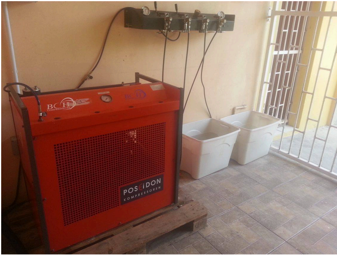
Figure 7 Air compressor recently installed at Sauteurs. Photo by Simone Kist, with permission.
