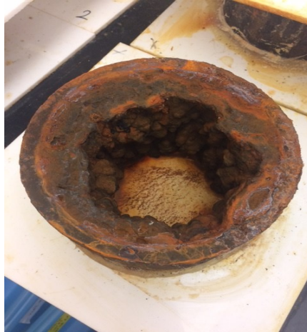
Figure 6.1 Harvested pipe section from a local distribution system.
