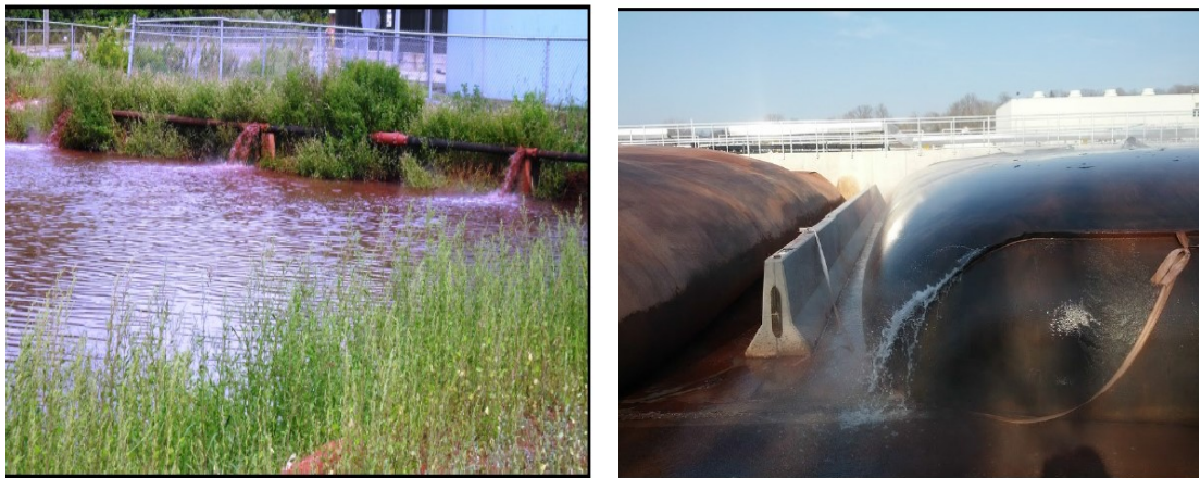
Figure 2-8 (a) Prior to Implementation of Geotube Units (b) Working in Operation after Geotube Installation (Bishop Water Technologies Inc. 2013)
