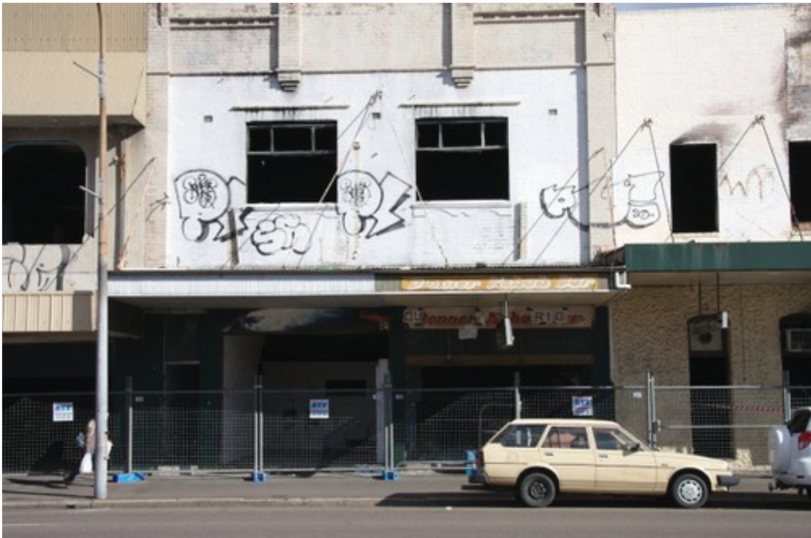
Newcastle Central Business District - Dilapidated storefronts; image from Renew Newcastle .
