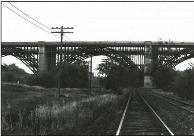
Fig. 6: View of viaduct from valley floor, illustrating elements identified as "point, line, and veil." (Photo: Morden Yolles)
