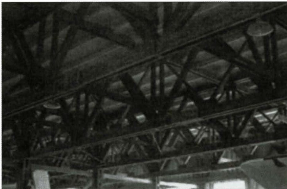
FIG. 11. BRANDON, MANITOBA. HANGAR NO. 1, VIEW OF SEVERAL REPAIRED TIMBER WARREN TRUSSES, SHOWING THAT REPAIRS ARE UNOBTRUSIVE AND DO NOT ALTER THE HERITAGE CHARACTER
