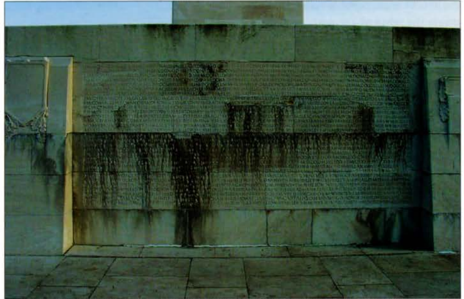
FIG. 6. DETERIORATION OF THE MONUMENT BEFORE RESTORATION. THE SURFACE OF THE MONUMENT HAD BEEN BROKEN UP BY A PATCHWORK OF DIFFERENT STONE TYPES, TYPOGRAPHICAL STYLES, CALCITE DEPOSITS, SURFACE DISCOLOURATIONS, AND SPALLING. | CABINET LEFÈVRE, MAY 2003.
