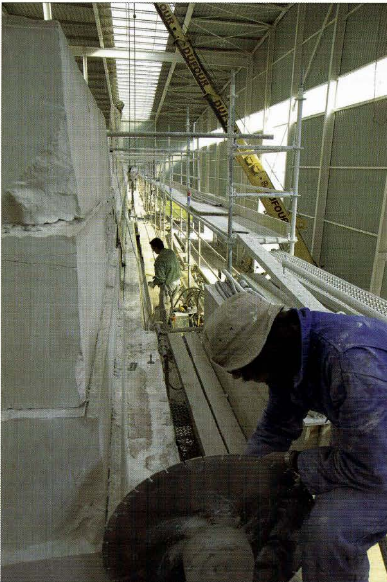
FIG. 1. DISMANTLING THE VIMY MEMORIAL: ROW AFTER ROW OF STONE BEING CUT AWAY FROM ITS CONCRETE BASE. | PHILIPPE FRUTIER, ALTIMAGE, FOR VETERANS AFFAIRS CANADA, JUNE 2005.
