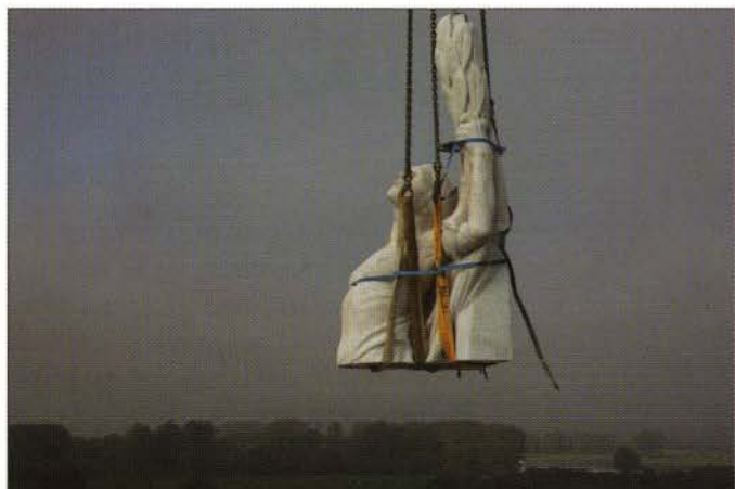
FIG. 2. PART OF THE STATUE OF PEACE BEING LIFTED OFF THE WEST TOWER, PRIOR TO REALIGNMENT AND REINSTATEMENT. | PHILIPPE FRUTIER, ALTIMAGE, FOR VETERANS AFFAIRS CANADA, OCTOBER 2006.
