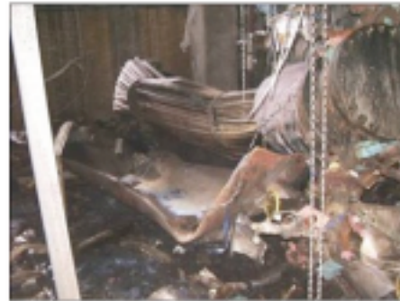
Heat Exchanger Rupture
