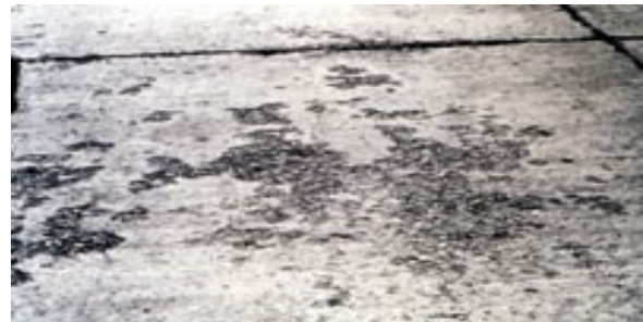
Figure 2.9 Concrete Scaling (PCA 2013b)
