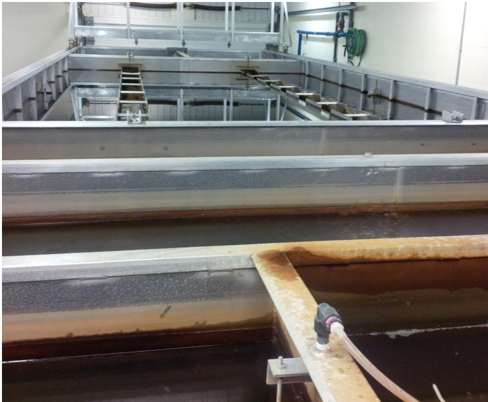
Figure 3.4: Rapid mix, flocculation, clarifier and filter tanks at the FWTP
