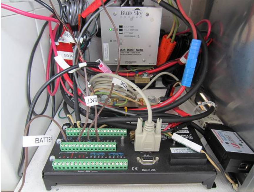
Figure 46: Experiment board (Including current shunt, charge controller and data logger)
