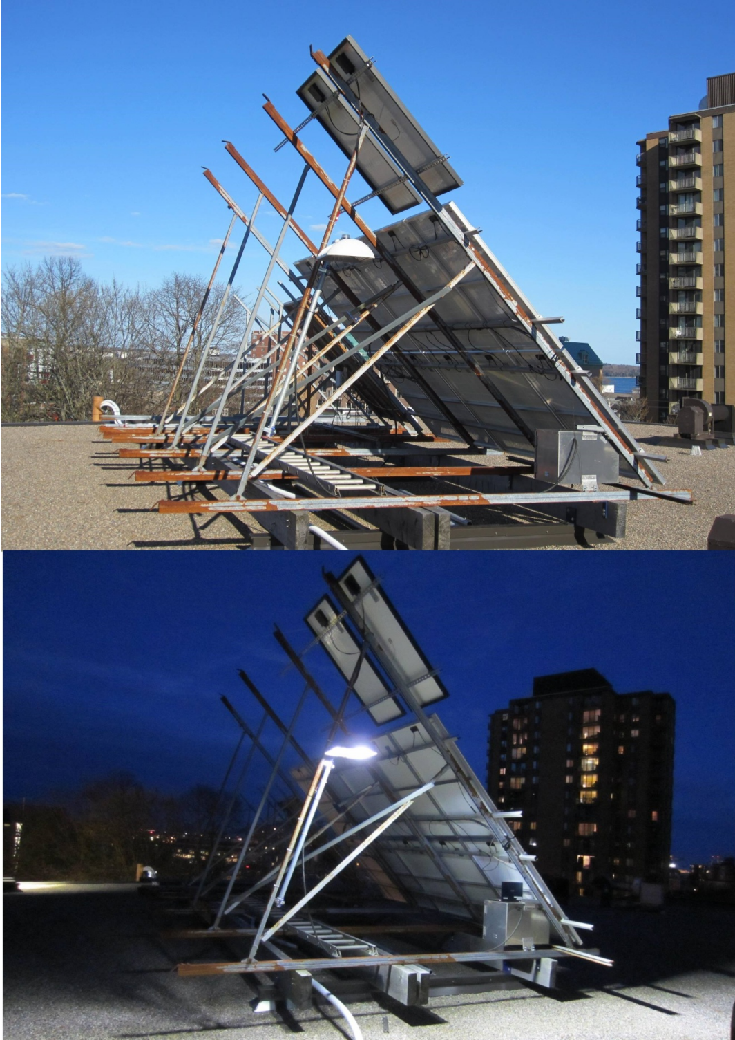
Figure 53: Solar street light setup (Day/Night)
