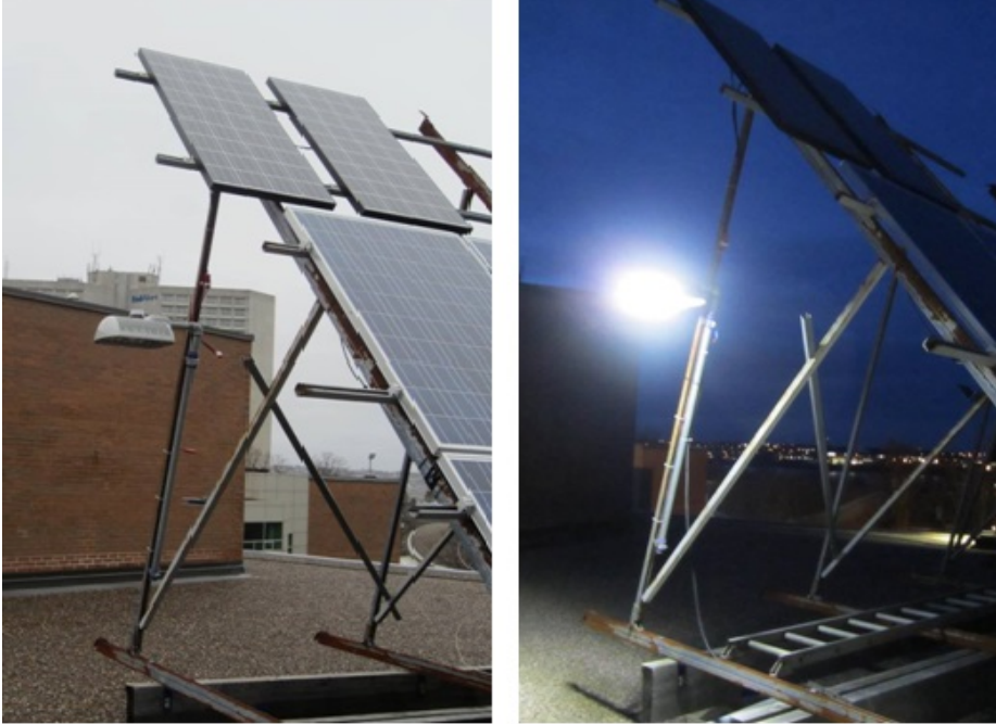
Figure 51: Installed street light (Day/Night)
