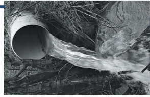
Unfiltered water flows out of outflow pipe
