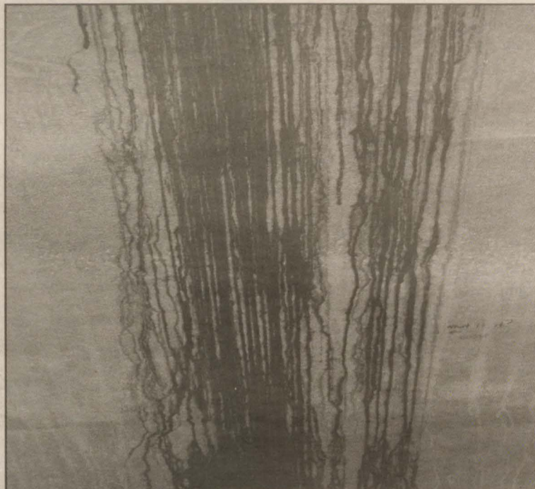
An unknown black substance is seeping from the basement ceiling of the Dal Arts Centre. / Photo: John Packman
