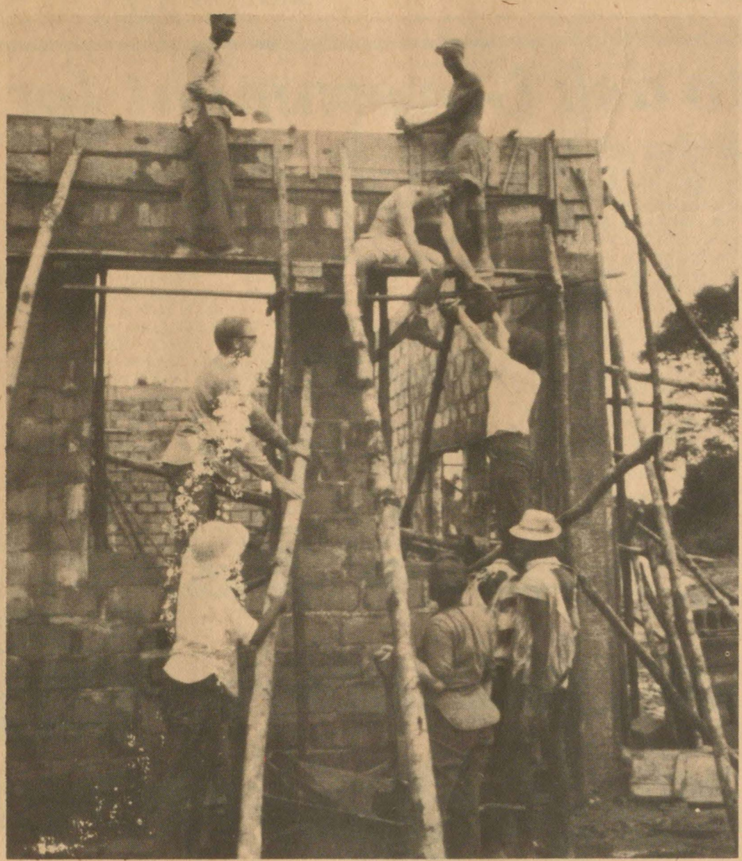
Crossroads and Liberians enjoy a cooperative effort to pour concrete for a tie-beam. Project was first of four buildings of a Y.M.C.A. camp being constructed at Nyeha, 45 miles northeast of Monrovia, the capital of Liberia. (Photo: JOAN ROBB)
