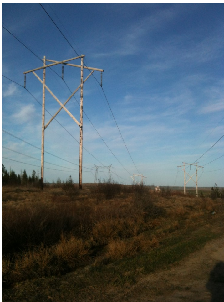
Figure 2.12: An example of Douglas fir transmission poles in service
