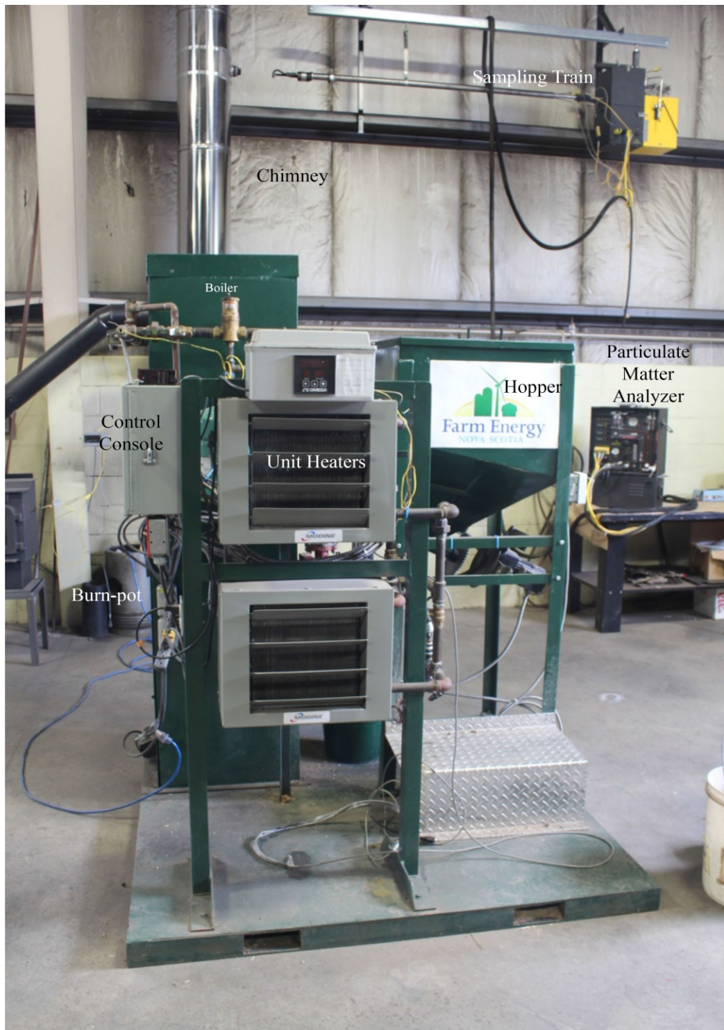
Figure 5. Agro-Pellet Boiler designed by LST Energy Inc., Pictou County, Nova Scotia.
