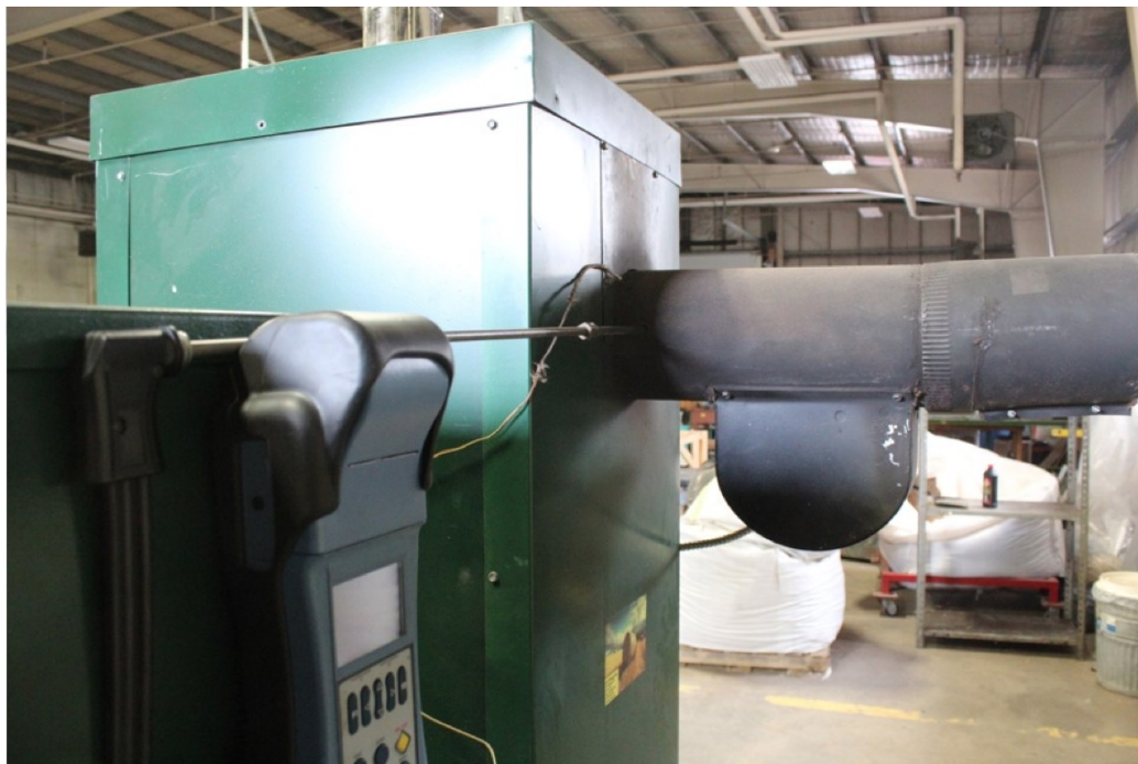
Figure 6. Eurotron Unigas 3000+ flue gas analyzer installed in the Exhaust of the Agro-pellet boiler.
