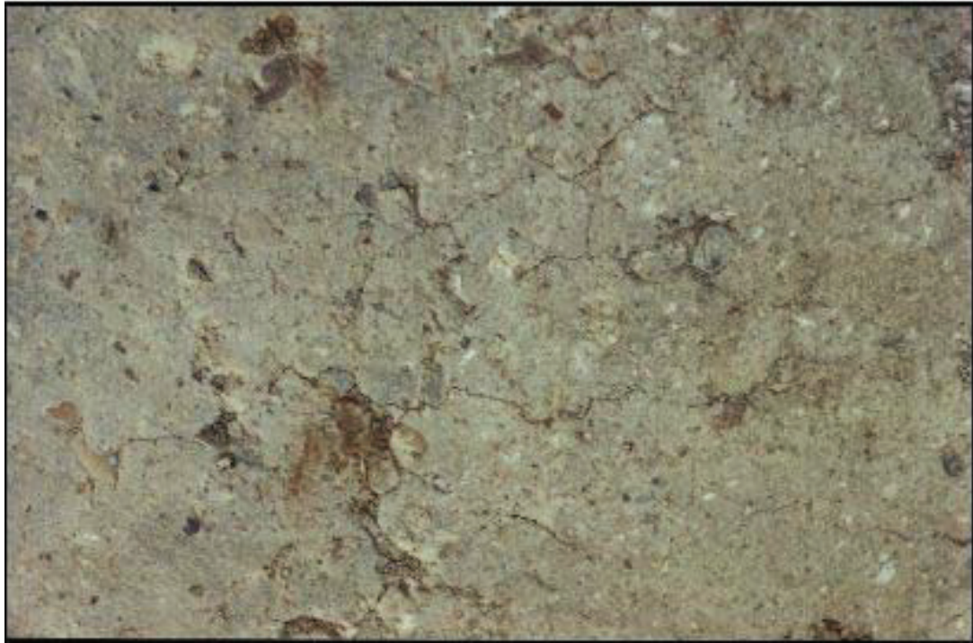
Figure 2-23 Cement treated material after microcracking (Sebesta & Scullion, 2004)
