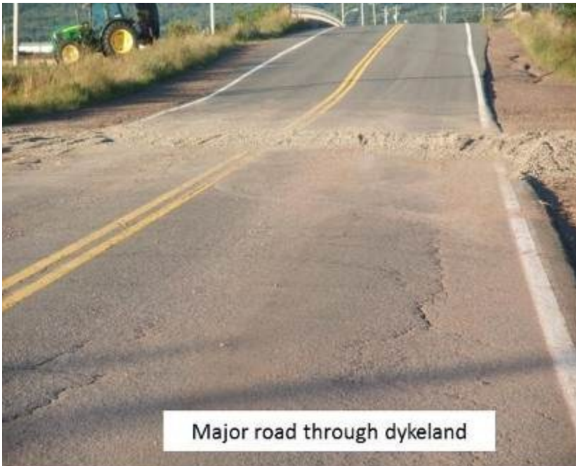
Figure 4.6: Damages caused by heavy rains in Central Nova Scotia, September 10, 2012
