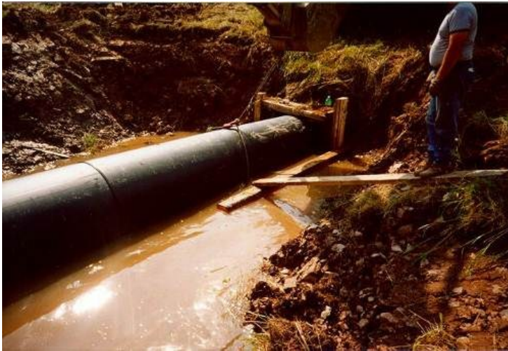
Figure 2.4: Modern aboiteau made of polyethylene plastic pipe (Source: Nova Scotia Department of Agriculture, 2007).
