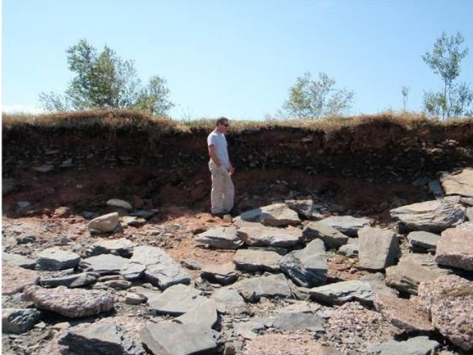
Figure 2.6: Dykes that require maintenance but are delayed due to lack of resources (Source: Post, G., 2011)
