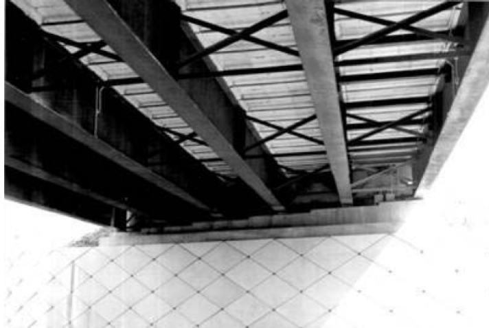
Figure 2.11 - View of the underside of the Salmon River steel-free bridge deck (Newhook & Gaudet, 2006)
