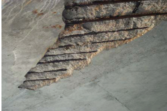
Figure 2.4 Damage in Marine Structure Showing Concrete Spalling and Corrosion of Reinforcing Steel
