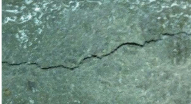
Figure 5.3 Maximum Plastic Shrinkage Crack Width in TER 50 Mixture
