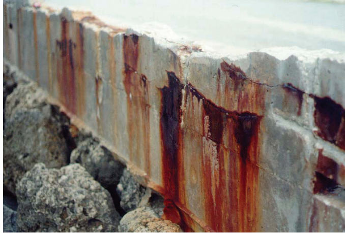
Figure 2.3 Corrosion Damage Exhibiting Rust and Cracking Parallel to Main Reinforcement
