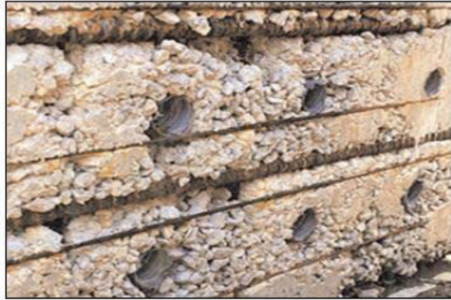
Figure 2.5 Segregation Due to Poor Compaction
