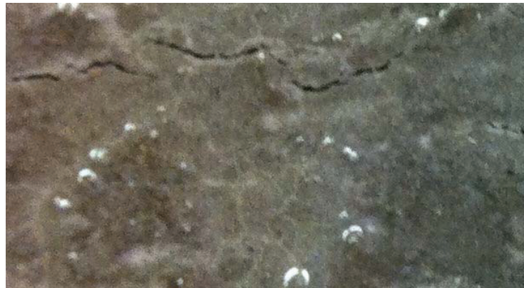
Figure 5.4 Maximum Plastic Shrinkage Crack Width in TER 50 with 0.20 % Fiber Volume Fraction
