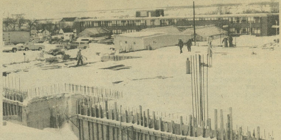
Construction work on the new library shows the basement storey and the commencement of structural work for the second floor.
