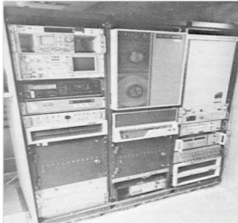
Figure 2-3: Equipment rack in mobile vehicle node of DSN [7].
