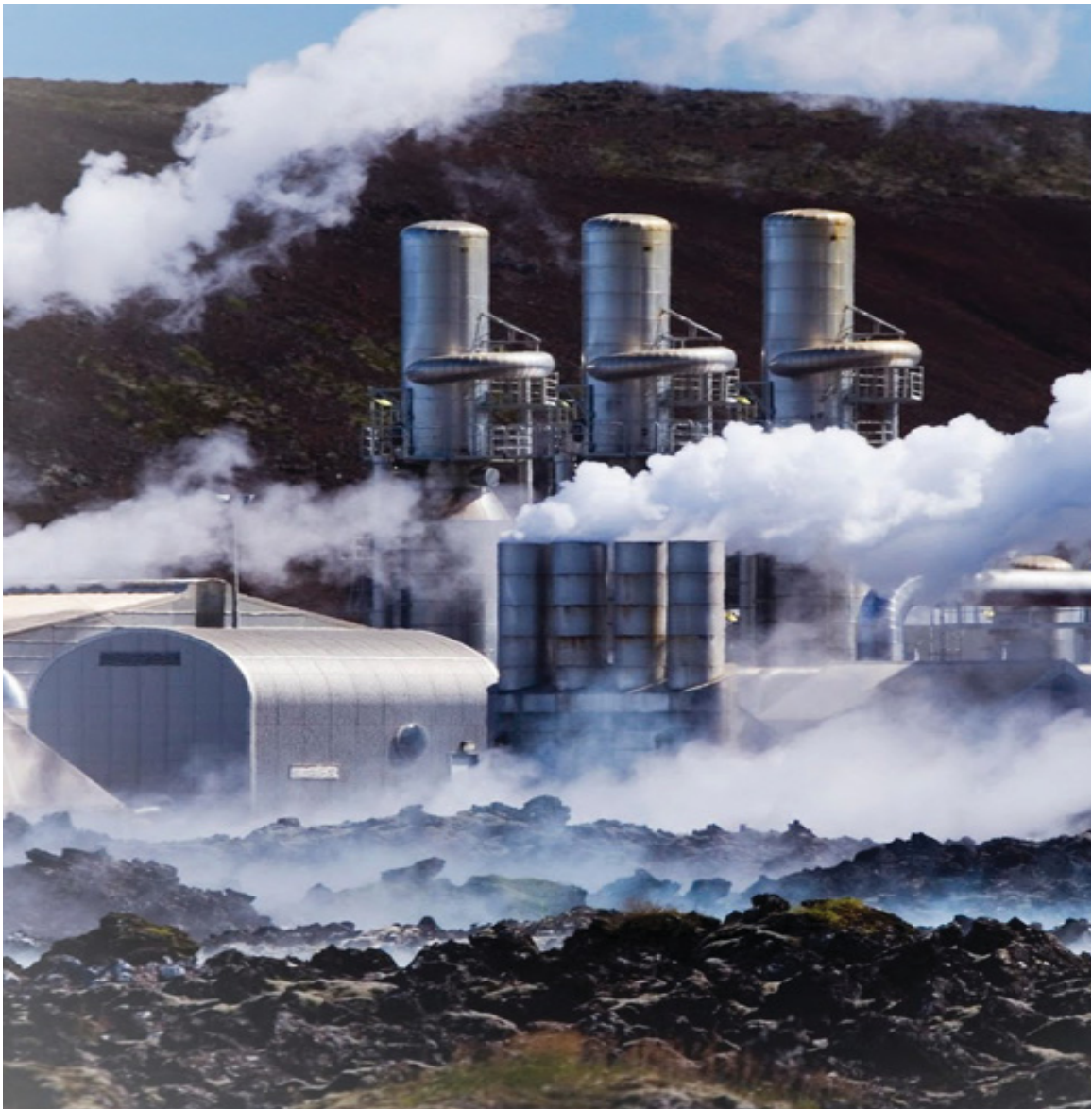
Svartsengi Power Plant and Blue Lagoon. From Terdiman, "Coder Corner."
