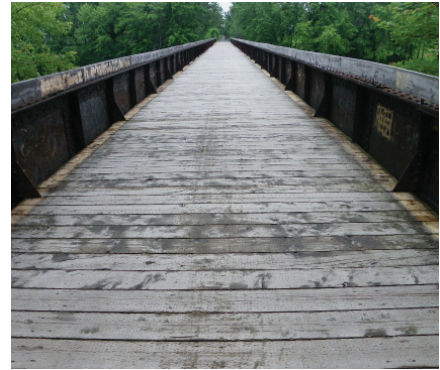
Wood deck of a former train crossing over the Nashwaak River, at its tributary towards the Saint John River.
