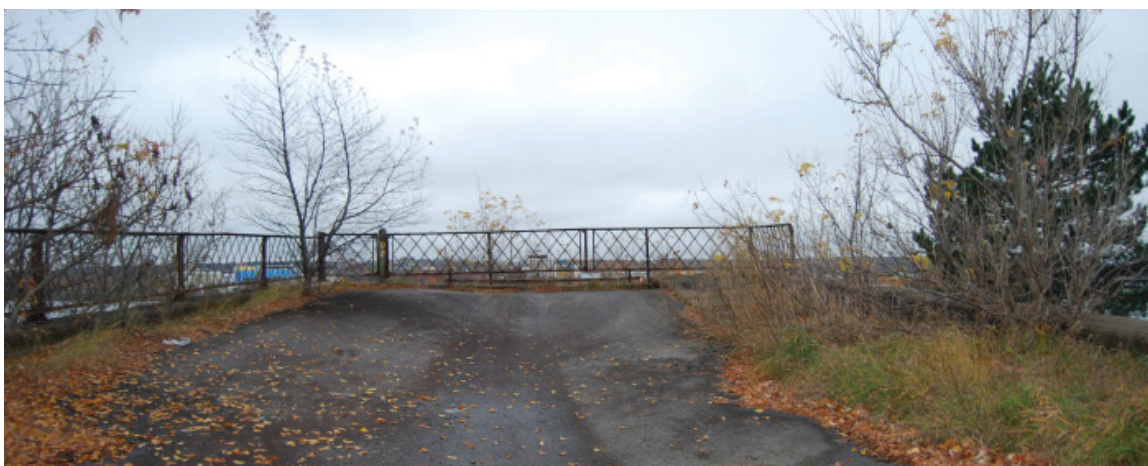
Overgrowth on Carleton Bridge ramp.
