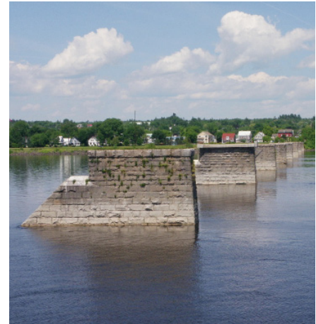
Existing piers from the former Carleton Street Bridge, as seen from the south side of the river looking towards the site.
